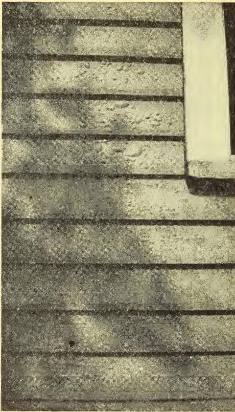
BLISTERING DUE TO MOISTURE IN THE WOOD
